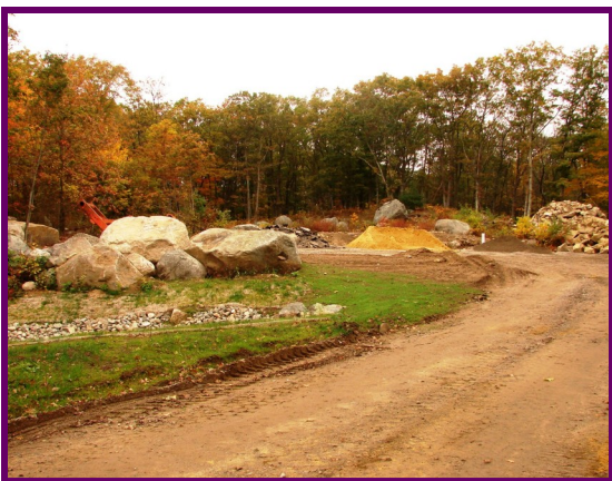
The site has been cleared and prepped for the construction of our new facility and parking lot (above).
