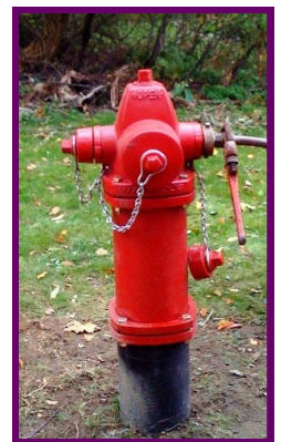
As site prep nears completion, a fire hydrant has been installed (above).
